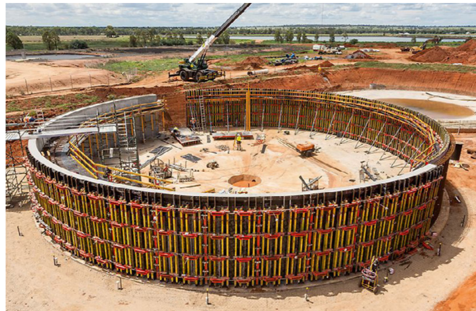
Dubbo Regional Council recently completed upgrades to its STP in order to keep up with expected population growth. Pictured, is one of the two clarifiers included in the upgrade.
