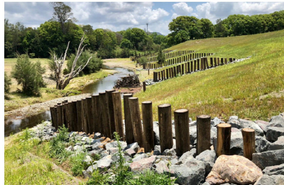
An example of river bank stabilisation along the Mary River in Kenilworth.
