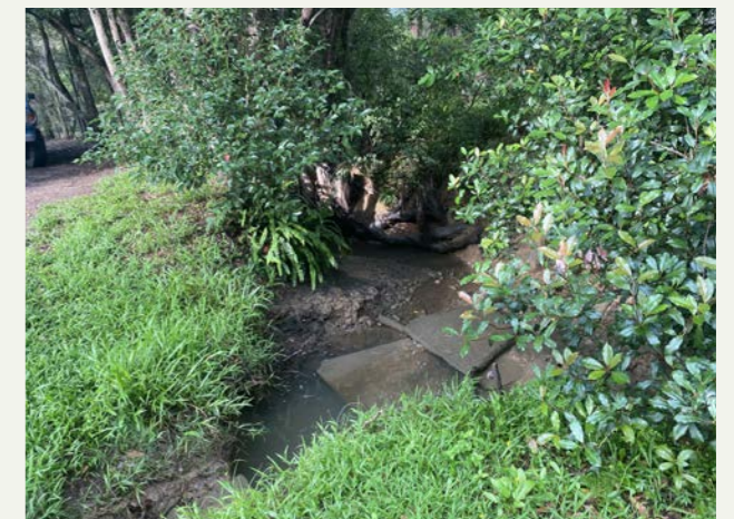
Heavily eroded and degraded drainage line
