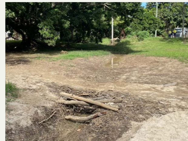
Existing drainage lines crossing the park areas. Image also shows silt deposit from the 2022 flood
