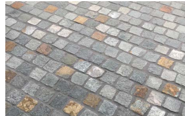
PEDESTRIAN THRESHOLD TREATMENT Note: the use of segmental pavers shall be minimal to ensure manageable on-going maintenance
