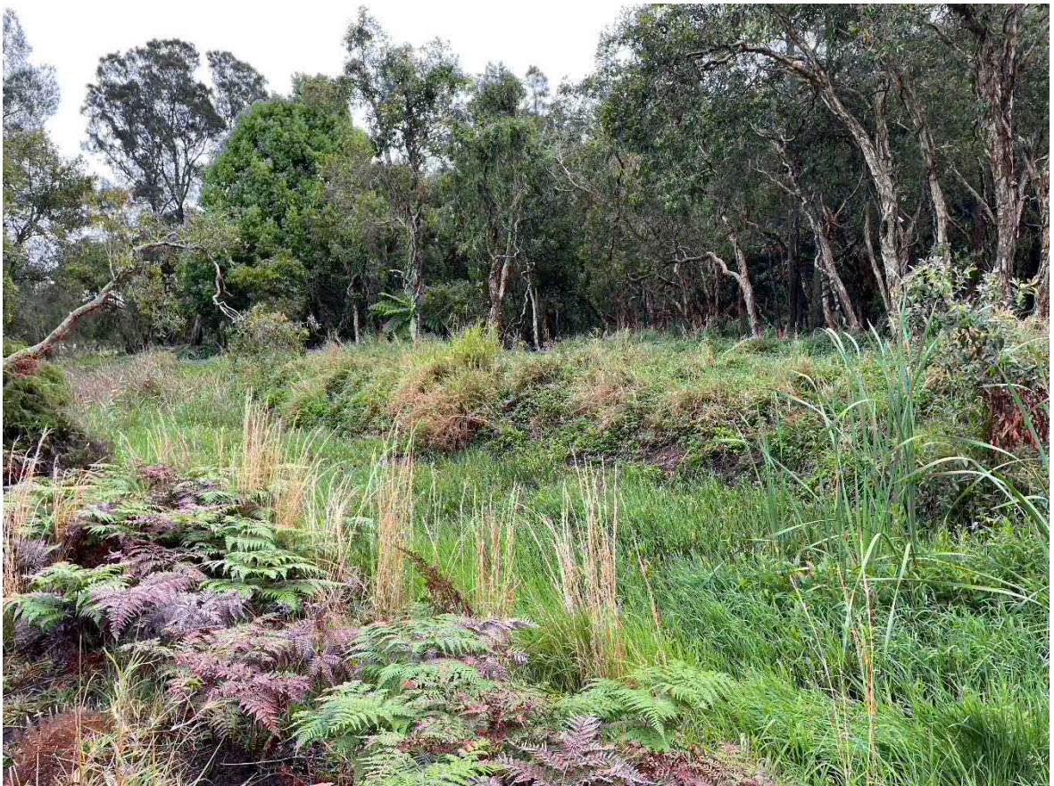
Figure 1-1 Existing drainage feature within the Sandhills Estate conveying untreated stormwater to Clarkes Beach
