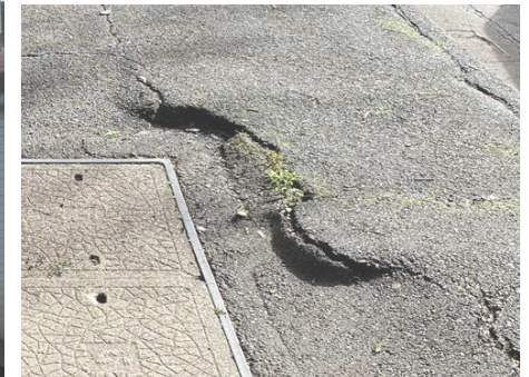
Roots lifting pavements causing trip hazards
