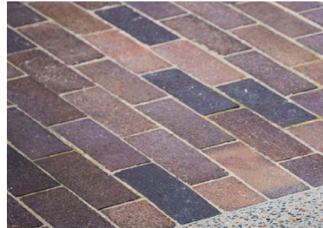
FOOTPATH - BRICK PAVING ON CONCRETE SLAB Type: Blue Mottle Paver Size: 225x75x55 Pattern: various Supplier: Lincoln Brickworks
