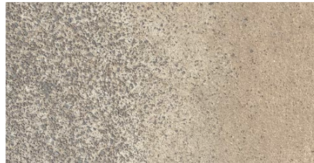
Concrete - weathered vs covered
