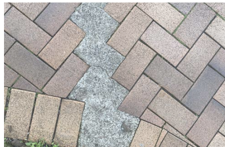
Brick paving with repair creating patchwork appearance
