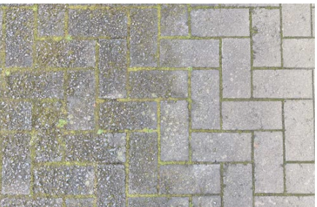
Brick paving - weathered vs covered
