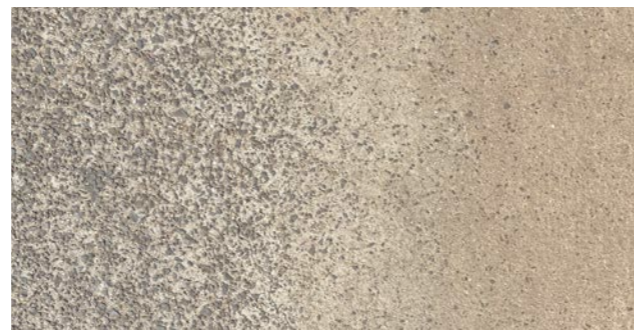
Concrete - weathered vs covered
