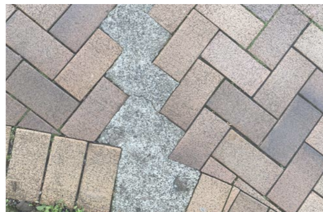
Brick paving with repair creating patchwork appearance
