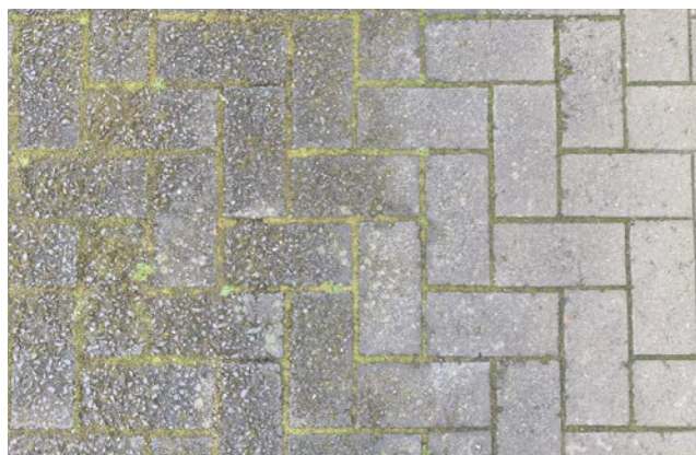
Brick paving - weathered vs covered
