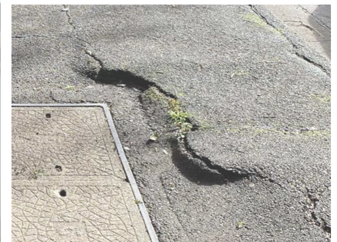
Roots lifting pavements causing trip hazards
