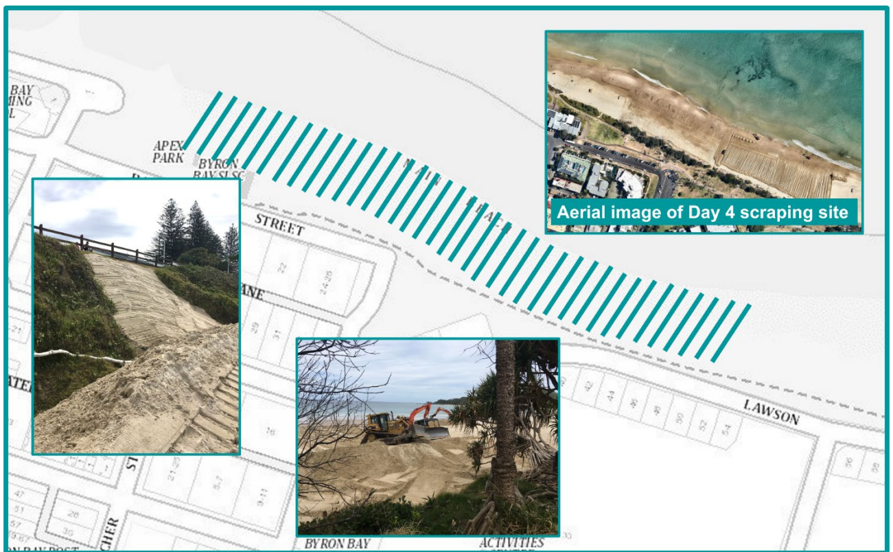
Figure 17: Day 4 (24/11/22) beach scraping works, opposite Byron Bay Surf Life Saving Club to opposite 50 Lawson St.
