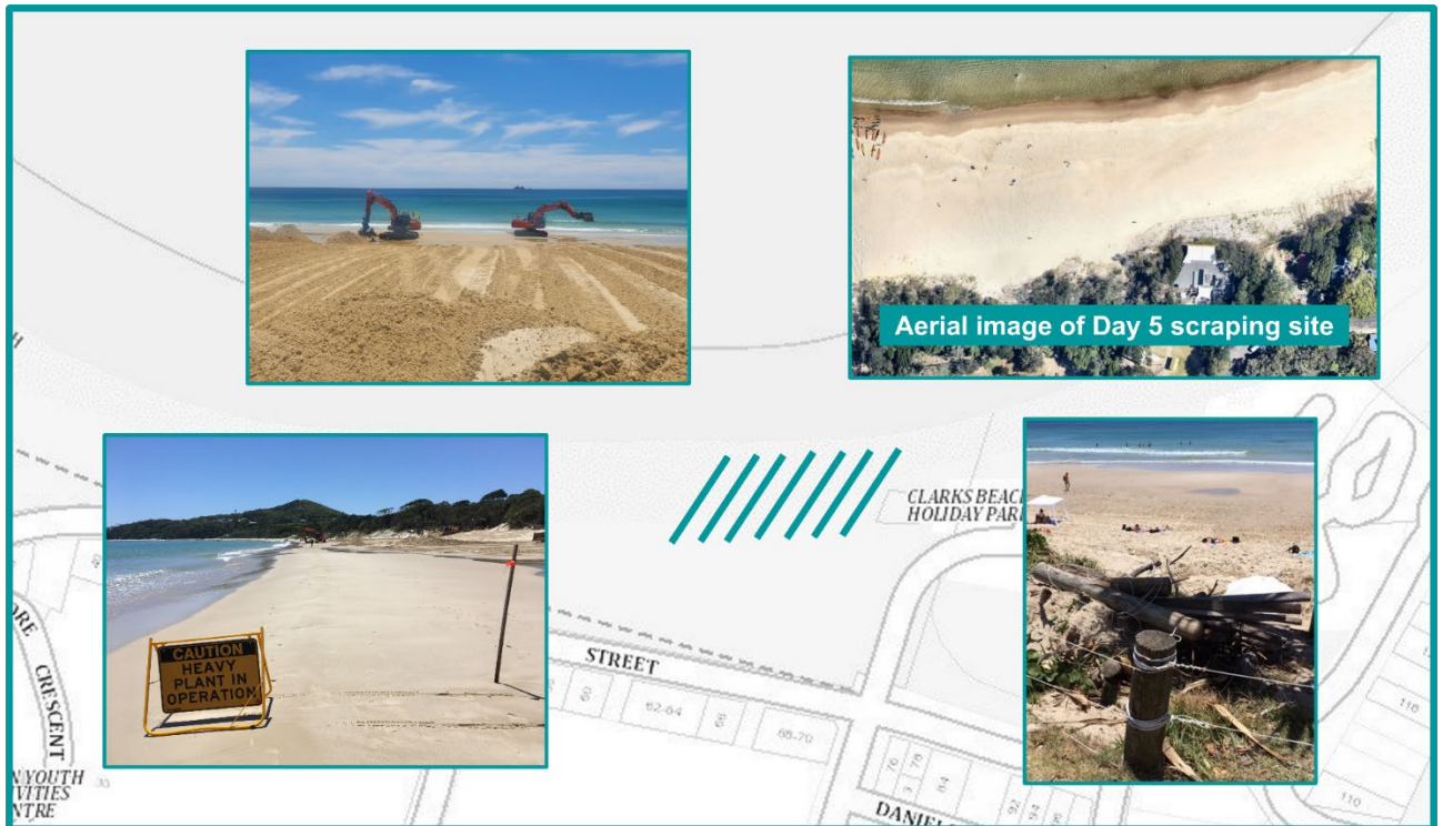
Figure 18: Day 5 (25/11/22) beach scraping works, located opposite 62-64 Lawson St to the Byron Beach Café.
