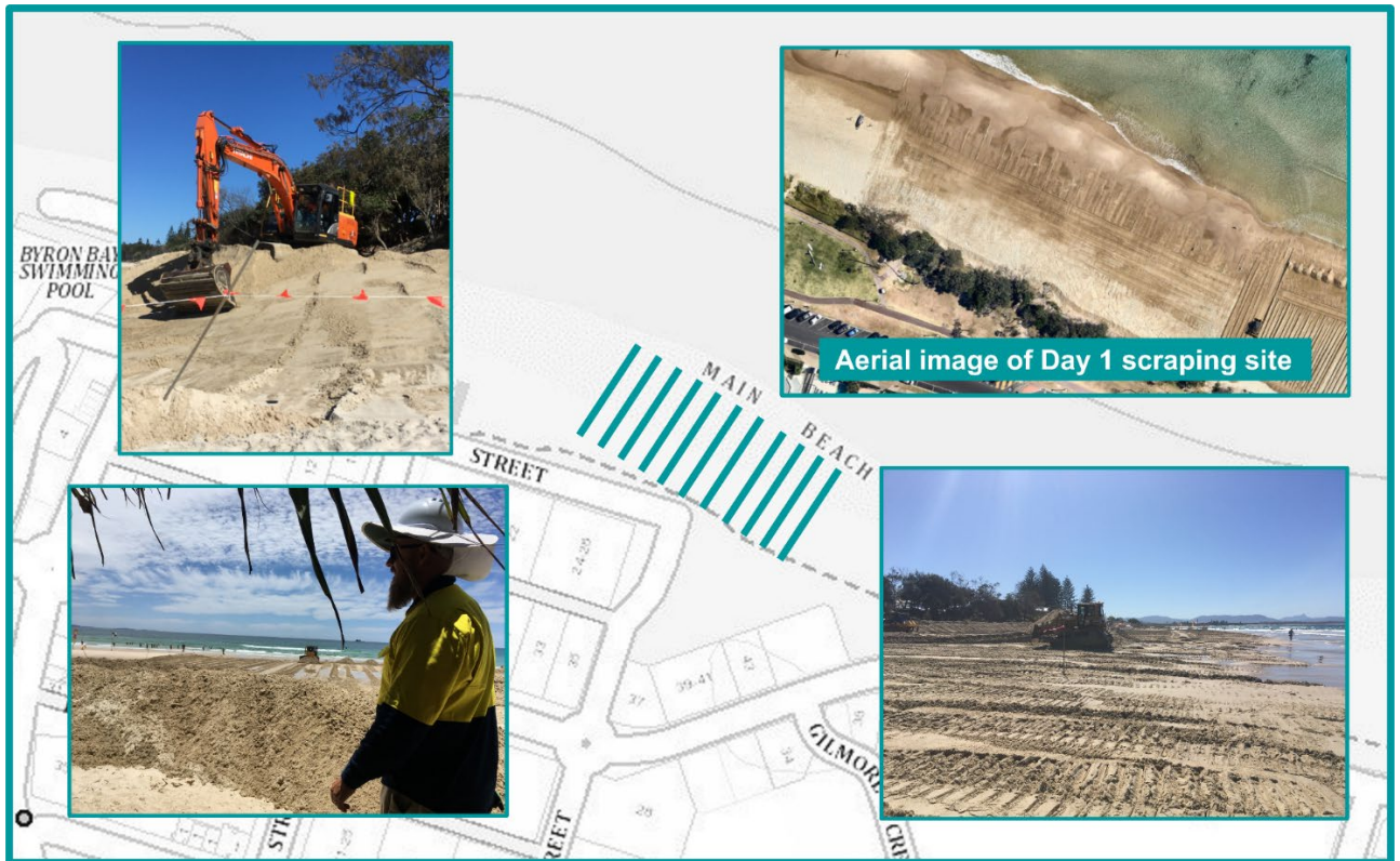
Figure 14: Day 1 (21/11/22) beach scraping works, located opposite 22 Bay St to opposite 43 Lawson St.
