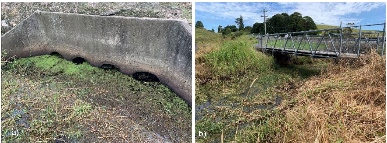
Plate 3: a) Culvert south of Ewingsdale Road within the Upper Union Drain (Moran's Hill) b) Footbridge over Union Drain downstream/ south of culvert.
