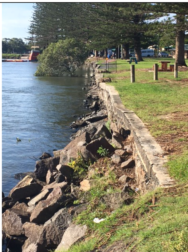
Photo - Si09 failing rock wall
