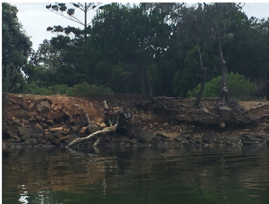
Photo – SI08 failing rock wall
