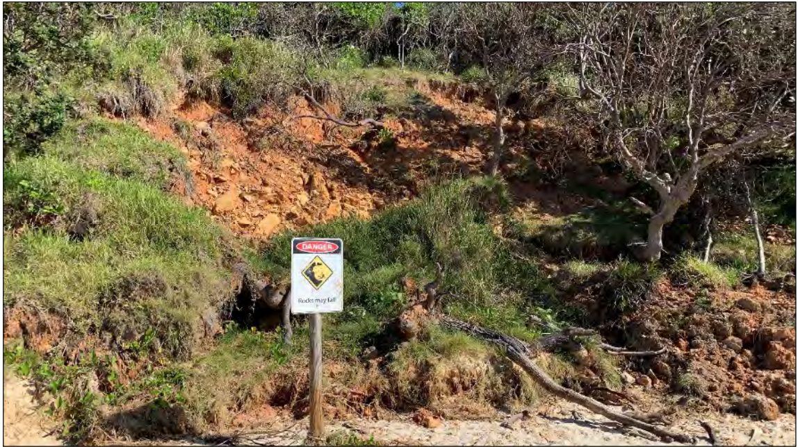
Figure 7: Looking southwest towards foreshore showing slumped area showing potential rock fall signage.
