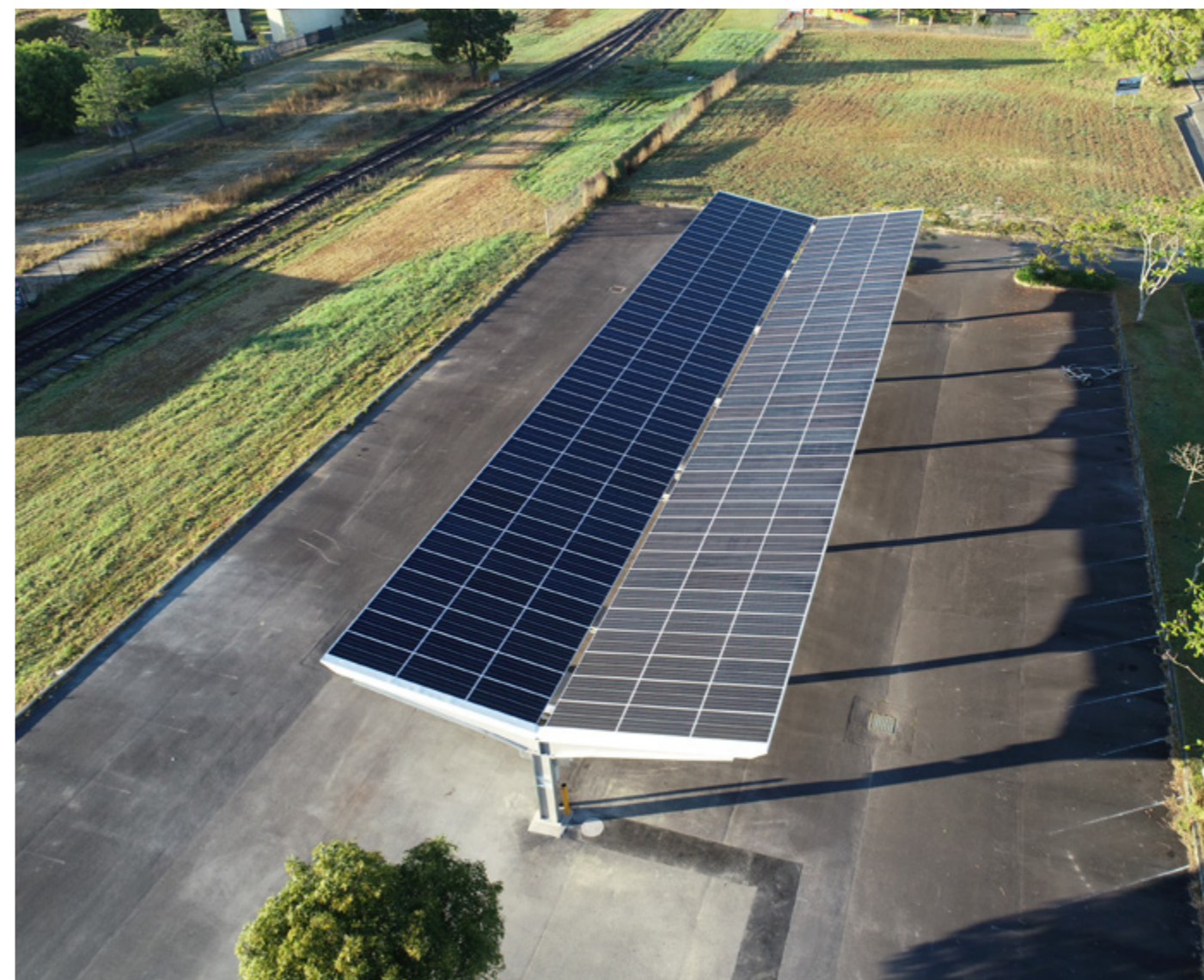
99kW solar carpark at the Council Administration Building, Mullumbimby.
