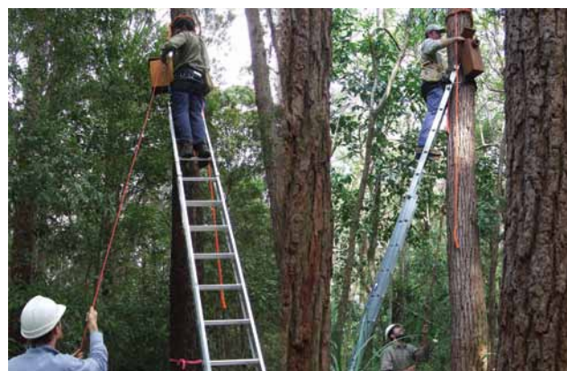
Nest boxes being installed using a sling and pulley system. Person on the ground can raise the box into position and hold it in place until it can be securely attached to the tree.
